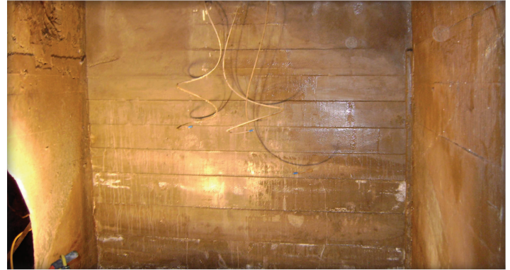
Formed Concrete Bulkhead with Injection Tubes
