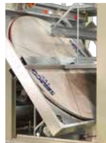
Energy Recovery Wheel
